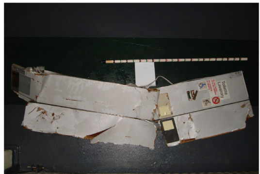
Figure 37: Metallic stiffeners deformed by buckling
