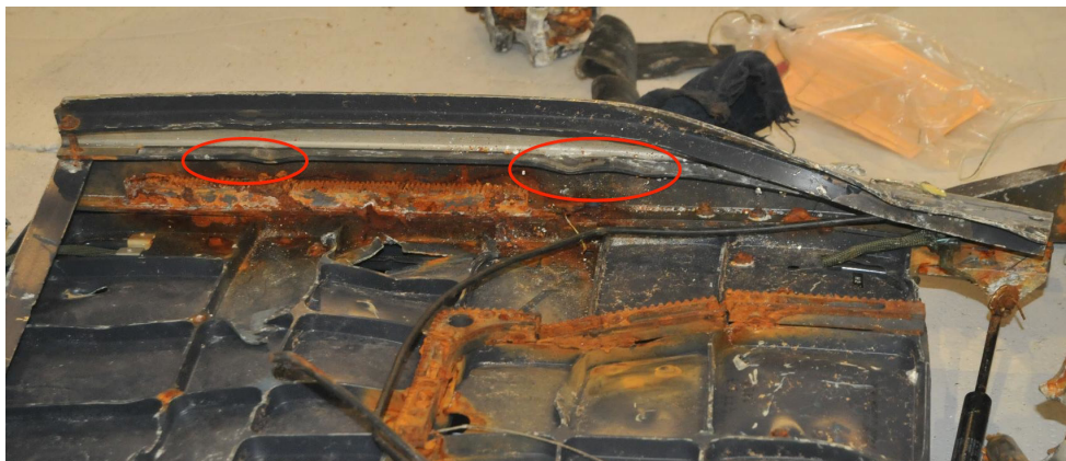
Figure 80: Roller marks on the guidance rail
